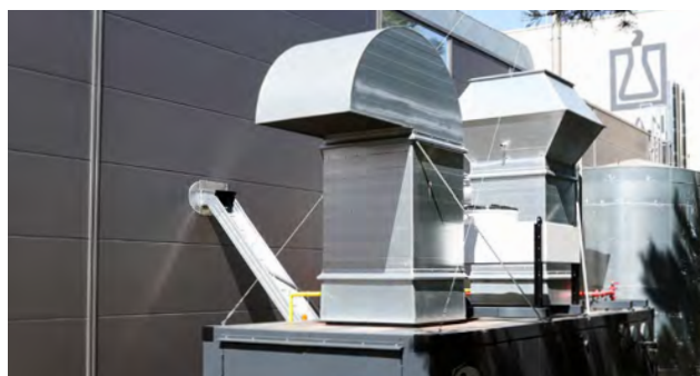
CHP station at BRAND KG
